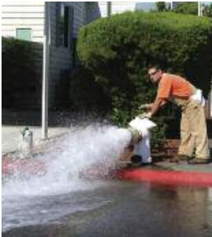
Public Works crew often flush fire hydrants to maintain water quality standards in Fairfield. Flushing is essential and should not be considered wasteful.
