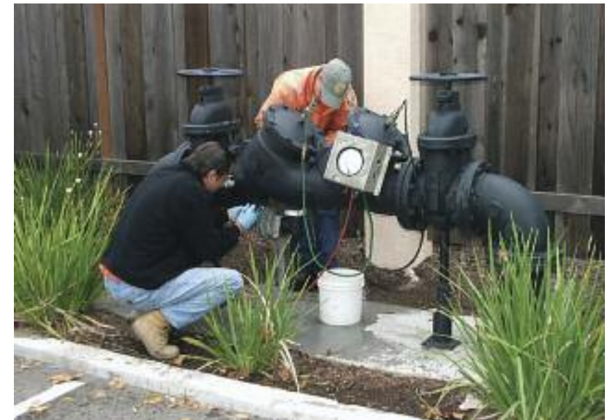
Public Works employees regularly check water pressure throughout the City.
